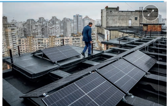
Valerii Pyndyk, head of a housing association board, on the roof of an apartment building where solar panels were installed in Kyiv, Ukraine, November 14, 2024. ALINA SMUTKO (REUTERS)
